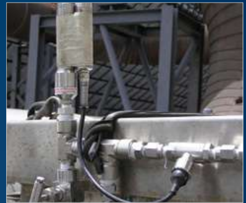
Water Pressure Monitoring
